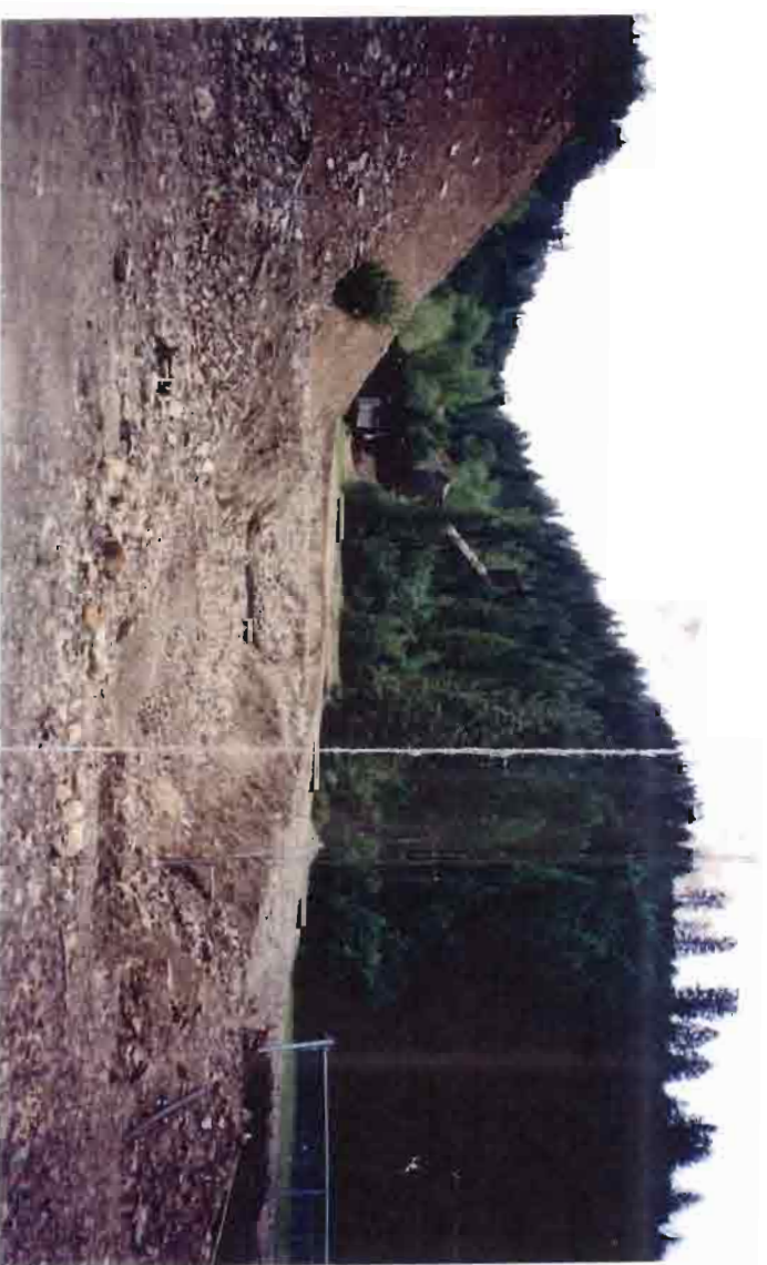
View of sediment fan at confluence of Nabob Creek. Culvert was clogged by large influx of sediment, and overtopped road.
